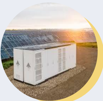
Battery Energy Storage System (BESS)
